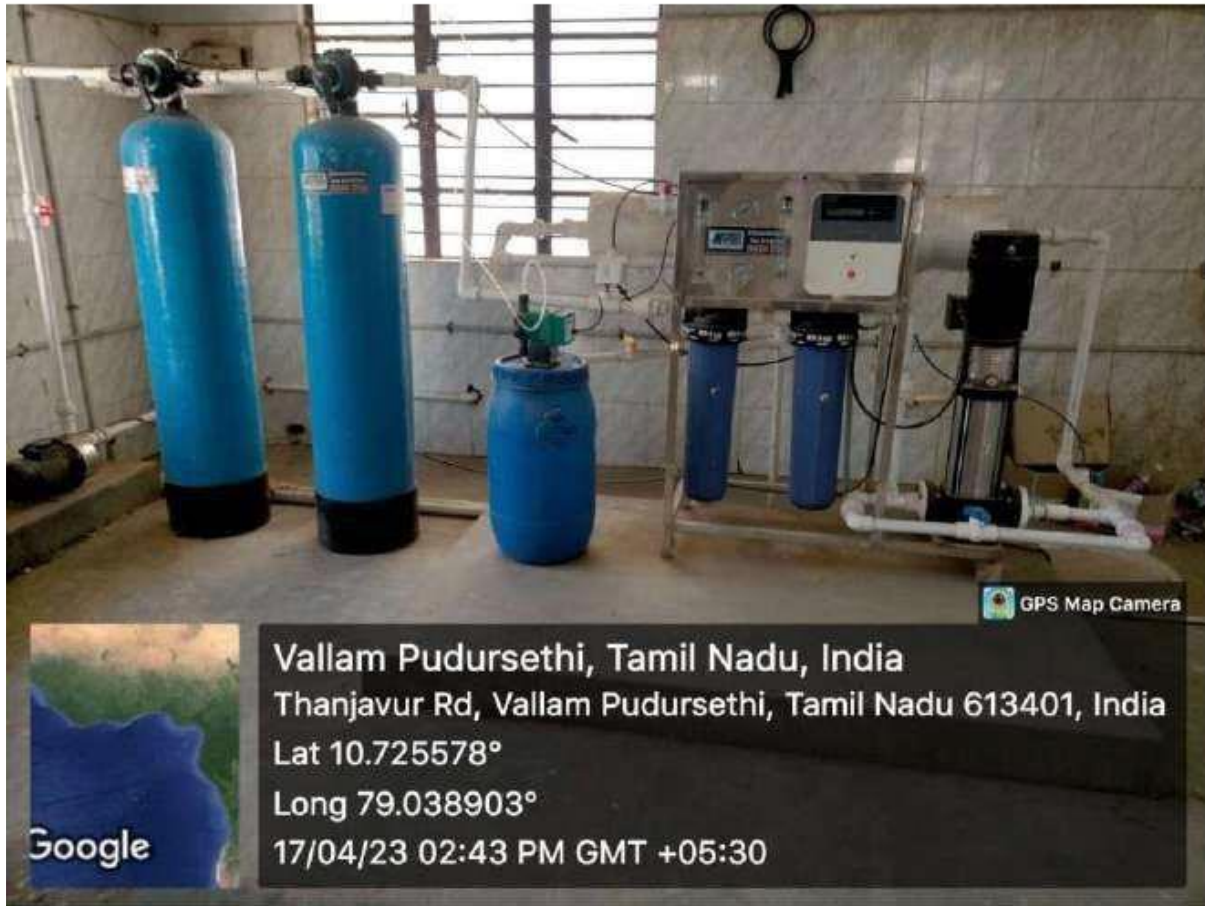
RO Central Control Unit in campus hostel
