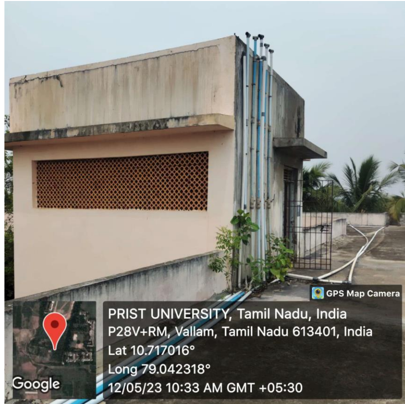
Water tank in Old Hostel
